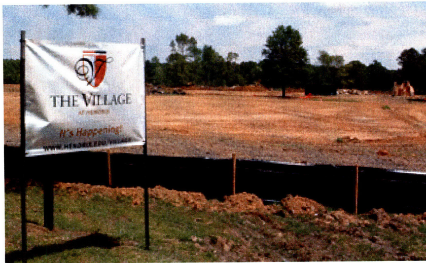
Figure 3.31: This photograph was taken in May 2008 and appears on The Village at Hendrix website with the note: "Preliminary street construction is expected to take place at The Village at Hendrix this week. Most of the clearing and grubbing of The Village site is completed. Crews are now expected to begin cutting the streets and performing backfilling, which will show the outlines of the streets inside The Village. Additionally, utility work at The Village is expected to begin by the end of the week. Area residents will now begin to see significant construction on the site." (Source: The Village at Hendrix website: http://www.hendrix.edu/village/ )
