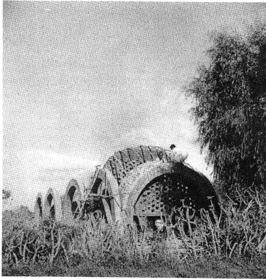
Figure 4.19. School under construction, Bavra, India. From Stephen Grabow, Christopher Alexander: The Search for a New Paradigm in Architecture (Boston: Oriel Press, 1983), 245.
