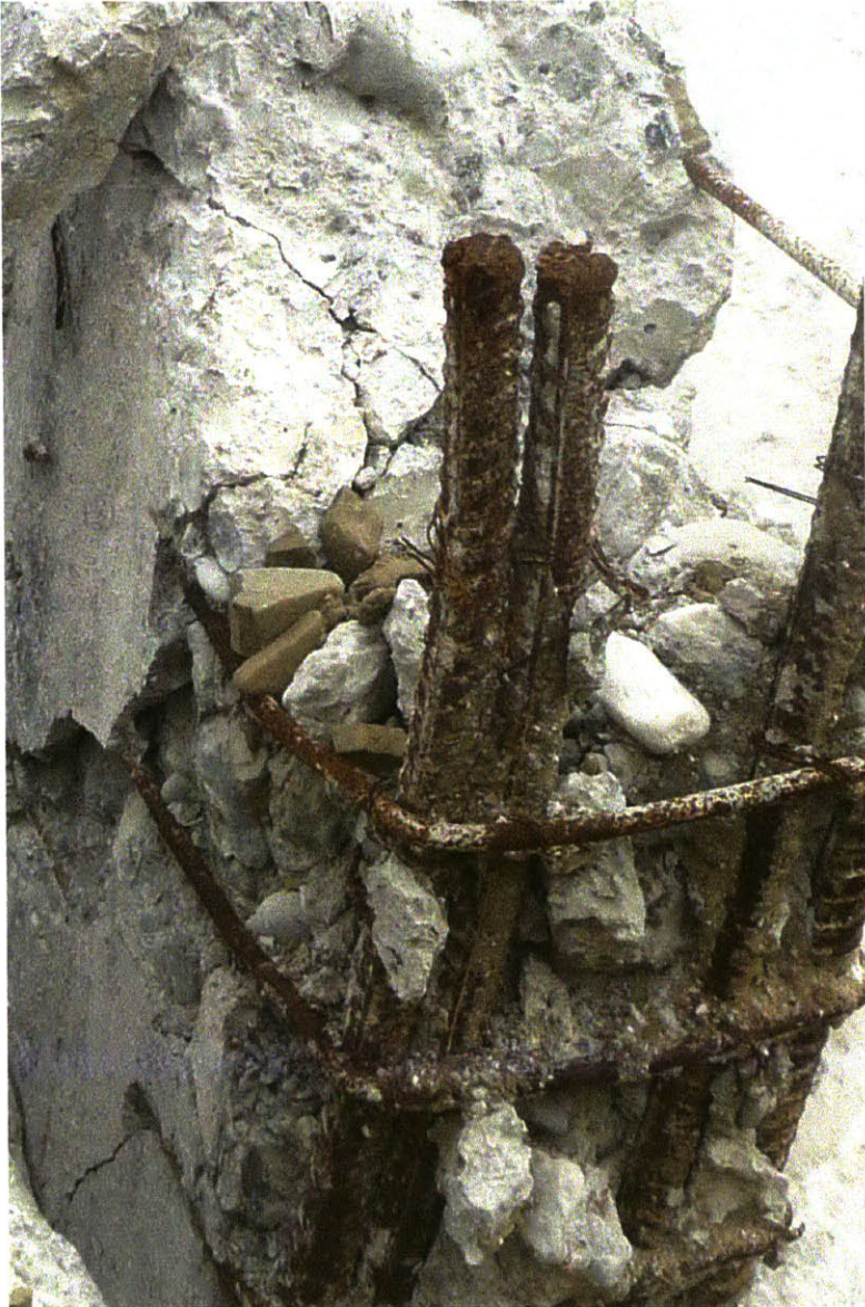
Beichuan School rubble, showing poorly graded aggregate in concrete
