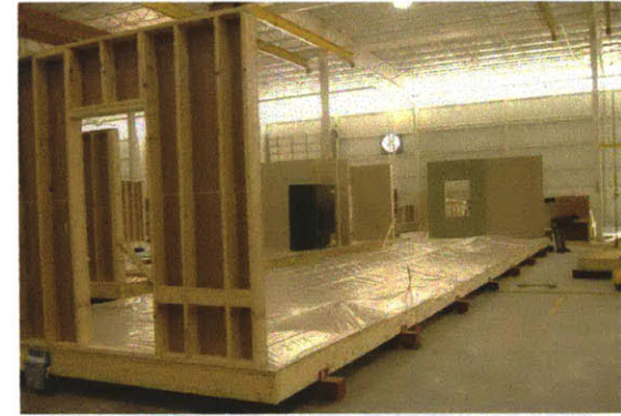
Penn Lyon Homes constructing a home module in their Selinsgrove factory (image: Penn Lyon Homes).
