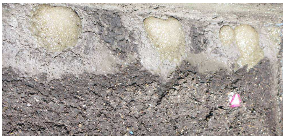
Figure 13: Scum Caked Gas Vents
