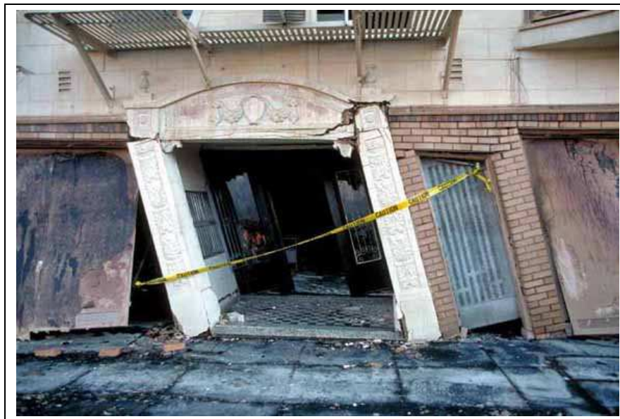
Figure 1-1: A partially collapsed building after an earthquake. [Photo credit: C.E. Meyer, U.S. Geological Survey]
