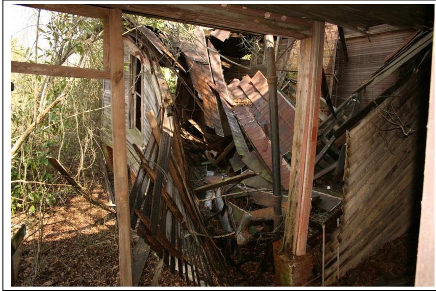
Figure 5-1: A room in a partially collapsed building. Flying in this room would likely be impossible with a 2D world model. [Photo credit: Sean Green. Picture taken of collapsing rural dwelling in Ora SC]
