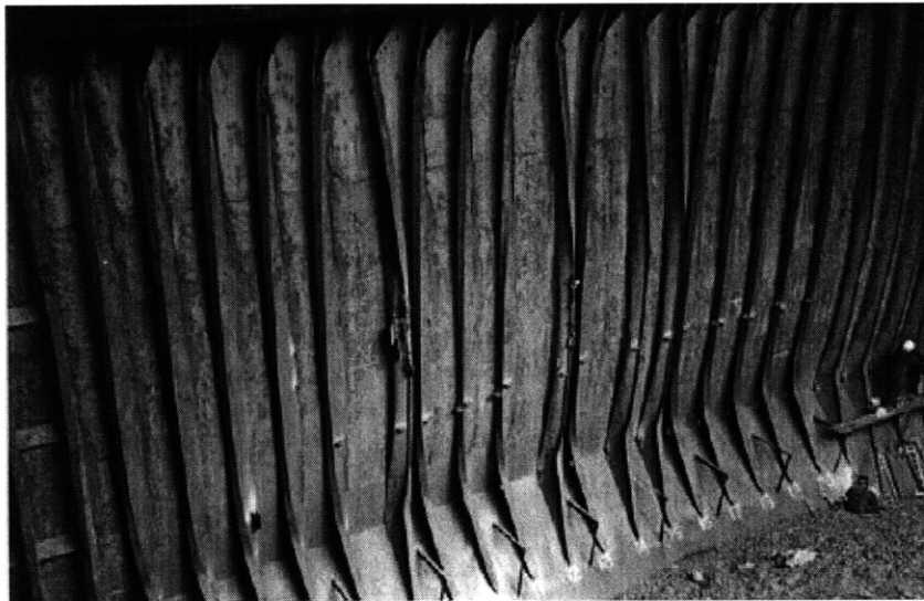
Fig 19: Deformation of Side Shell Frames Under Global Deflection
