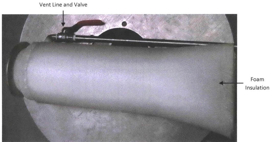
Figure 4-48: Container with Vent Line and Insulation
