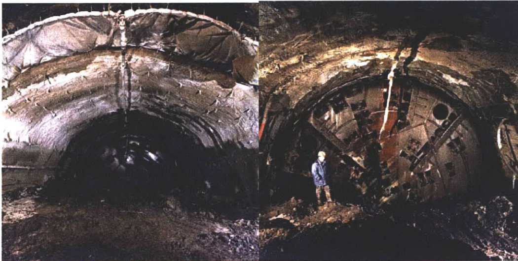
Figure 3.75 Access chamber completed with the TBM in the background (Barla and Pelizza., 2000).
