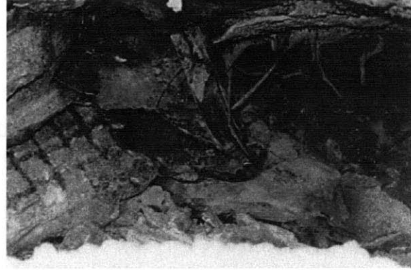
Figure 3.31 Failure of the support in the Bolu tunnel (Elmalık right tube) at km 54 + 135 (Dalgıç, 2002).
