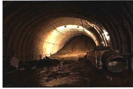
Aspect of the front after collapse (Ingress of soil and water)
