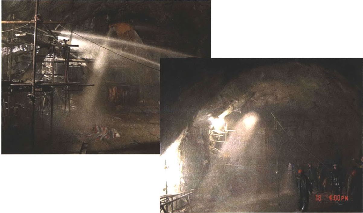
Figure 3.26 Water burst resulting in flooding, China (private correspondence)
