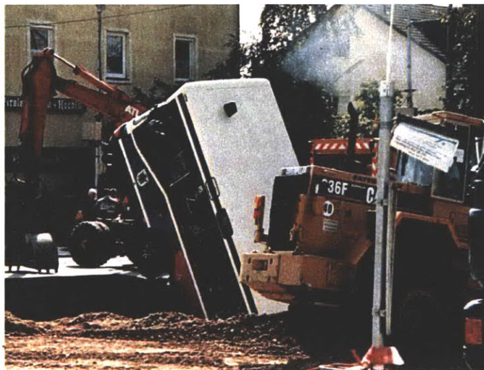
Figure 3.18 Crater caused by a collapse of the subway tunnel in Munich, Germany, 1994 (Wannick, H., 2006)
