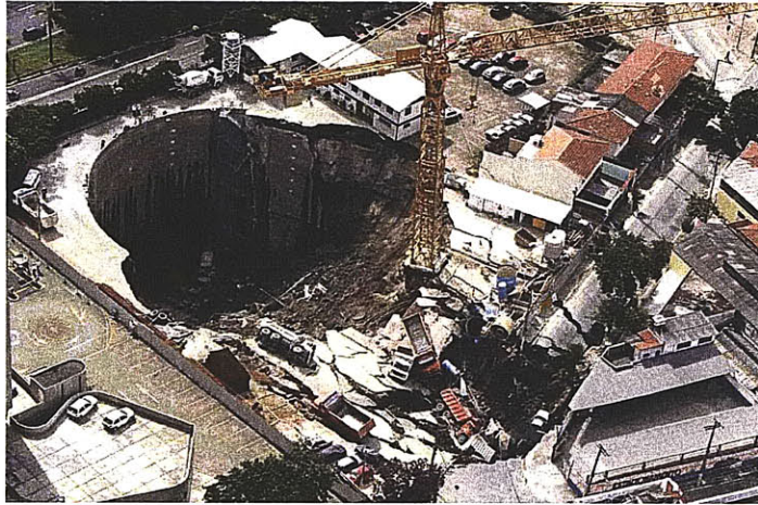
Figure 3.19 Collapse that occurred in Pinheiros Station, São Paulo, Brazil, 2007 (Barton, 2008)
