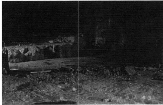
Figure 3.32 Invert squeezing in the Bolu tunnel (Elmalık left tube) at km 64 + 260 (Dalgıç, 2002).
