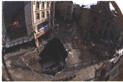
Collapsed area at the surface
