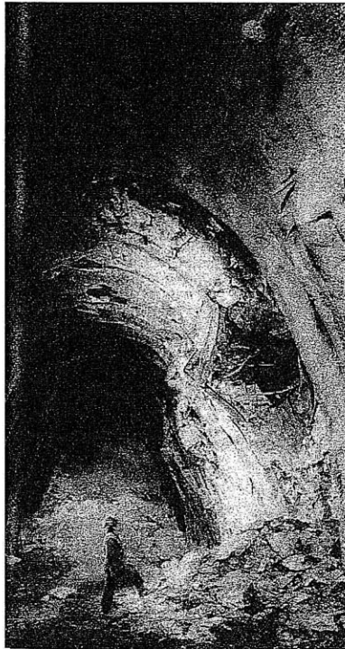
Figure 3.29 Picture of deformed primary lining due to swelling clays, Naples, Italy (Wallis, 1991)
