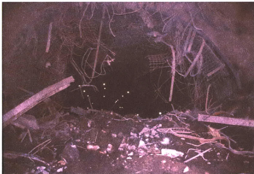
Figure 3.16 Partial collapse at Gotthard Base tunnel, Faido section (Einstein, 2007)
