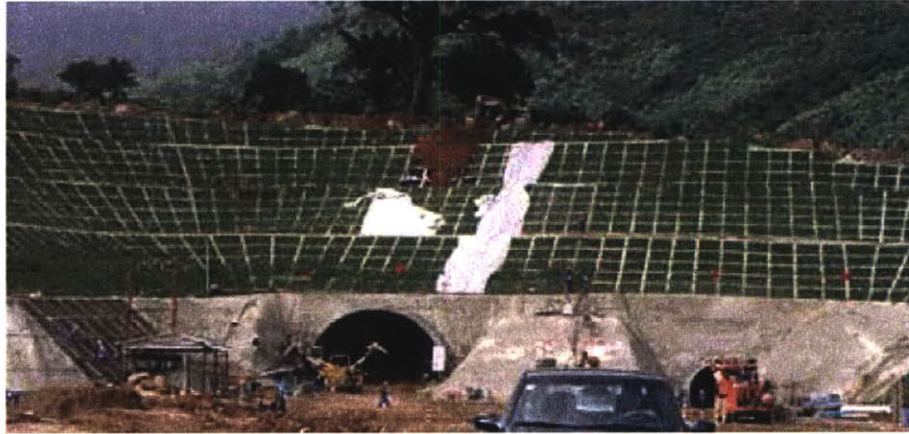
Figure 3.35 Cave in of the South portal slope in the Haivan tunnel, Vietnam (Fukushima, H., 2002).
