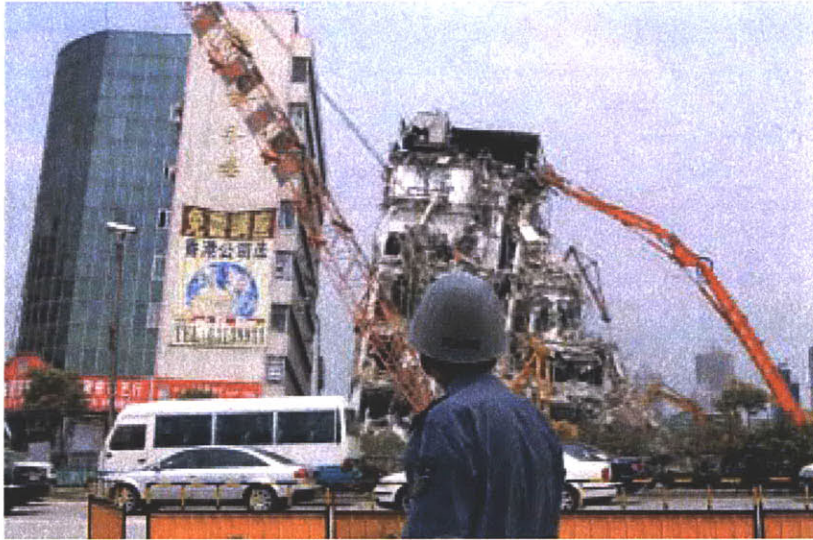
Figure 3.21 Demolition of buildings after the tunnel collapse in Metro Line No. 4 in Shanghai (Munich Re Group, 2004)
