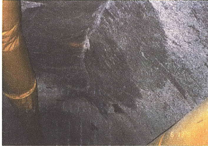
Figure 3.27 Rockburst at the crown in a in a waterway tunnel in Korea (Lee et al., 2004)
