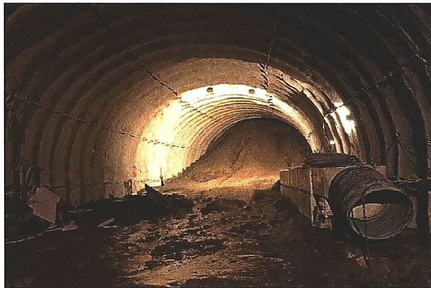
Figure 3.25 Aspect of the front after collapse (ingress of soil and water), Lausanne, Switzerland (Stallmann, 2005)
