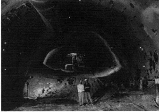
Figure 3.30 Heave in the Bolu tunnel (Elmalık right tube) at km 54 + 135 (Dalgıç, 2002).
