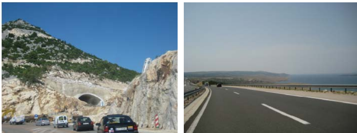
Figure 19: New road under construction , new road reaching to the Adriatic below Split
