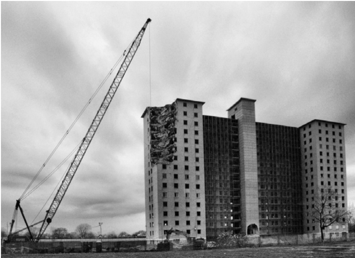
Figure 1.1: The Demolition of Chicago's Robert Taylor Homes (Image Source: Flickr user chicagoeye)
