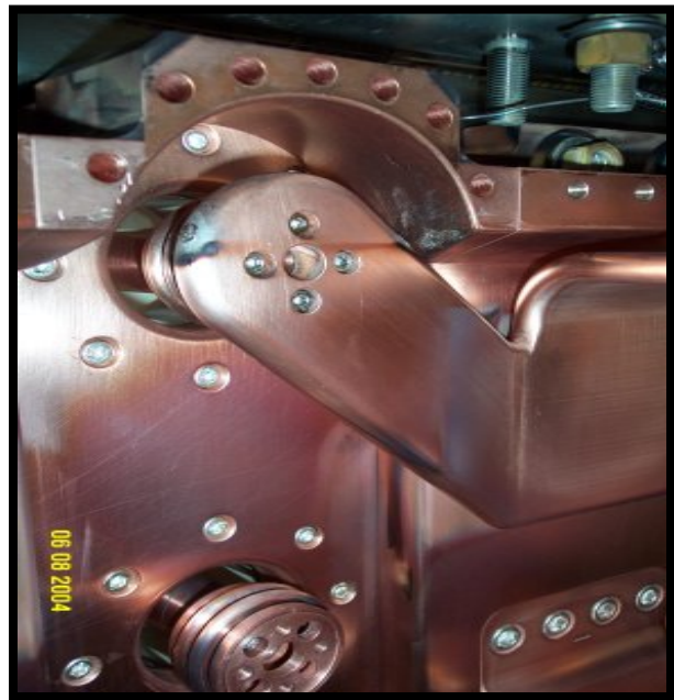
Fig. 9 Evidence of breakdown in feed system
