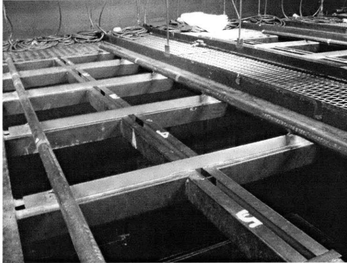
Fig. 4: The grid, including lighting pipes, of the Loeb Experimental Theater
