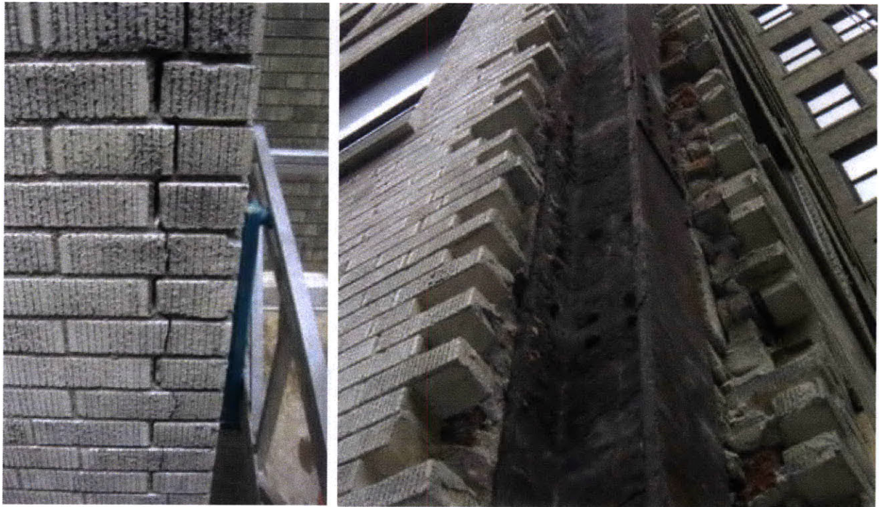
Figure 6: Cracked Masonry due to Differential Expansion and Rust-jacking of Embedded Steel Column
