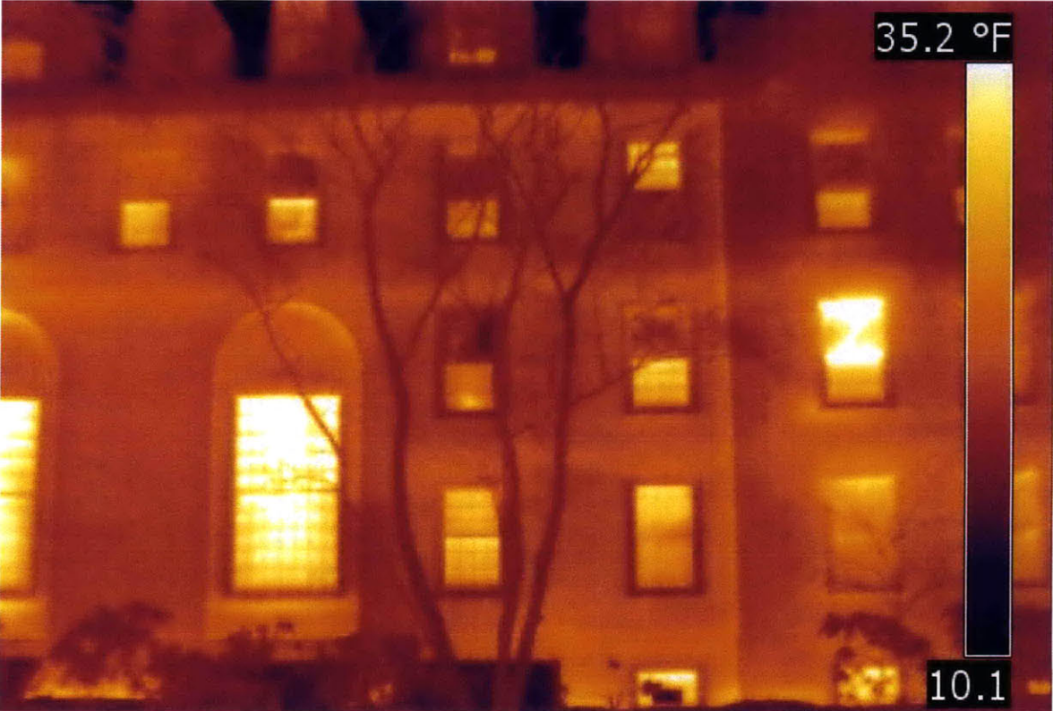
Figure 45: Infrared Thermogram Source: Hathaway, 2010
