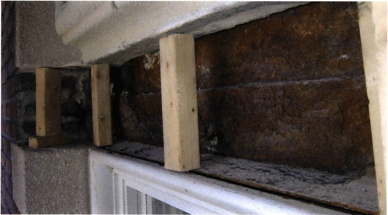
Figure 7: Deteriorated Secondary Structural Framing
