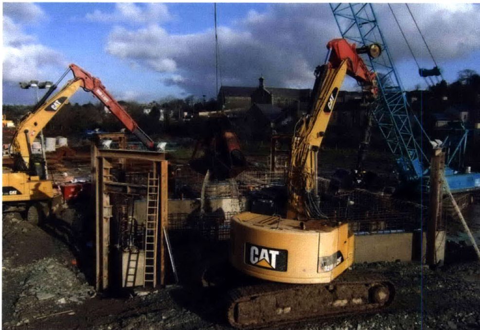
Figure 2-21: Sinking of main pump station caisson using various excavators and hydraulic jacks
