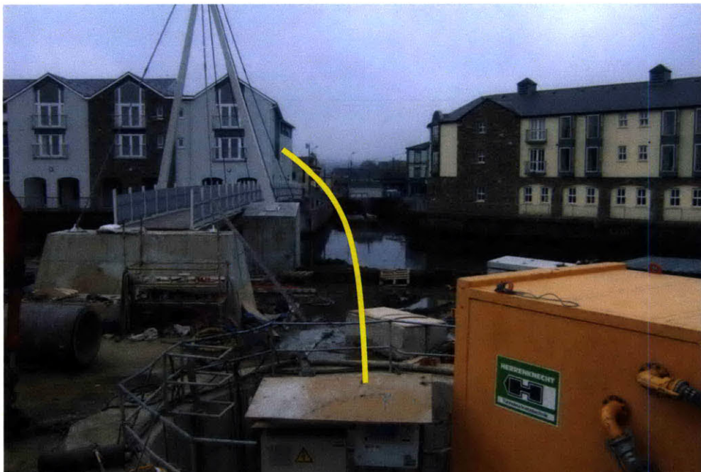
Figure 2-27: Tunnel alignment: (a) schematic (blue line is tunnel), (b) photograph from launch shaft
