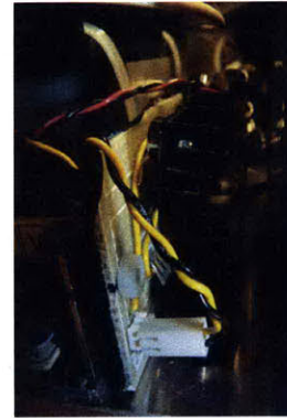
Figure 3-9: Voltage regulators and heat sinks.
