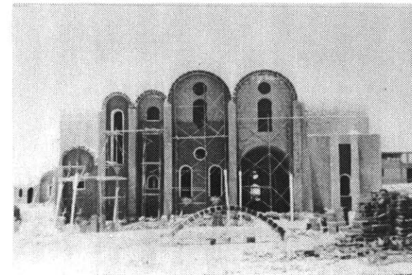
Fig II.10: A view of one of the houses during construction. Five months were all that were needed to reach this stage. One square meter of built area is costing exactly half the price of a similar residential type house using the conventional system of construction.
