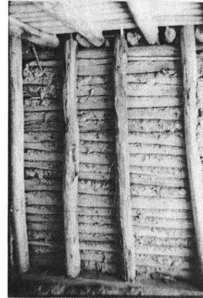
Fig II.14: Back of a wall and ceiling which shows the wattle-and-daub construction.
