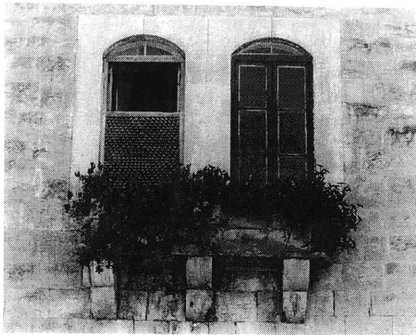
TWIN WINDOW DETAIL FROM MAROUF ABU-CHAKRA'S HOUSE IN DOWNTOWN BAAQLINE. THE TRADITIONAL CLOISTRA IS STILL IN USE.
