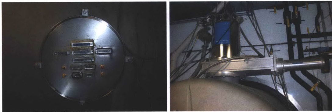
Figure 4-57: Areas of the vacuum chamber that leak. (left) A feedthrough plate with poorly-installed D-subminiature connectors. (right) A gate valve beneath the cryogenic pump.
