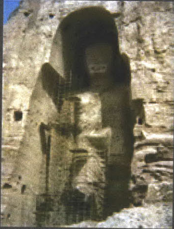
Repairing/preserving the broken leg and arm of the west Buddha. The missing or damaged pieces of the Buddha were reconstructed with similar materials. They also tried to implement reinforcement efforts, so it was not purely a cosmetic effort to repair the damages.
