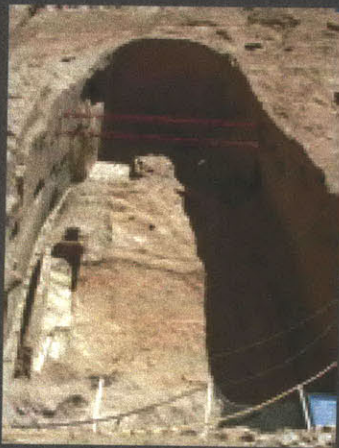
Latest efforts to salvage the niches, with cross bracing to keep the walls of the niches from falling down.
