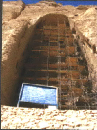
Repair efforts after the bombing, in 2004, where the niches were filled with scaffolding to brace the vulnerable state.
