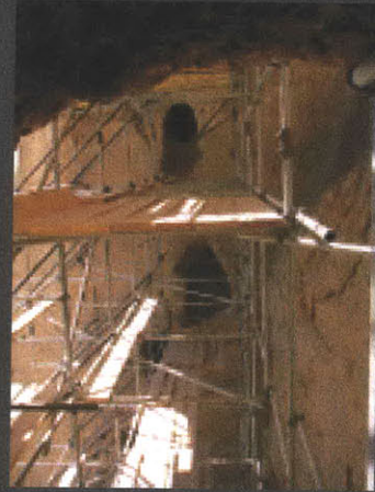
Repair efforts after the bombing, in 2004, where the niches were filled with scaffolding to brace the vulnerable state.
