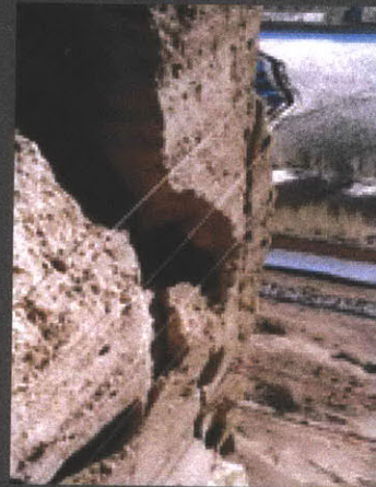
The niches are held together with wire cables at points of massive vulnerability, in an effort to keep the large pieces from falling over, which would most likely result in the collapse of the niche.
