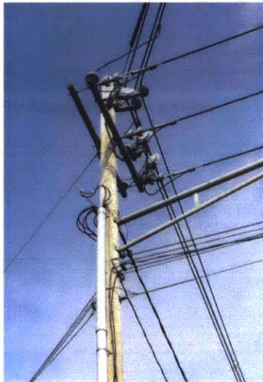
power lines as network
