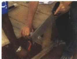
Cutting PVC pipe to the right size (Pipe held in place with a wrench)
