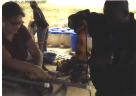
Drilling holes through the PVC pipe. Drill goes straight through the PVC pipe so in the end, there are holes every 90 degrees around the pipe (easier done with a vice)
