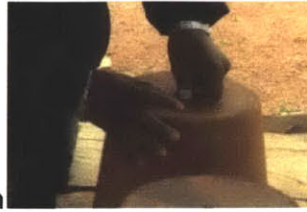
Sanding the hole to be large enough for a 3/4" PVC pipe to fall through
