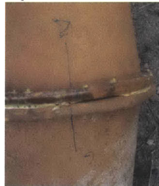
Figure 46 Gaps in the Seal Due to Lack of Gorilla Glue Expansion
