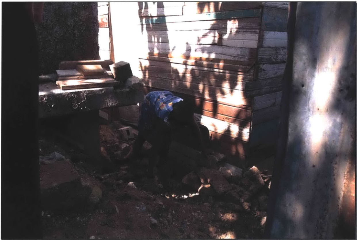
Figure 2: Woman building retaining wall around foundation of her house. Port au Prince, March 2011. Photo courtesy of Daniel Weissman.
