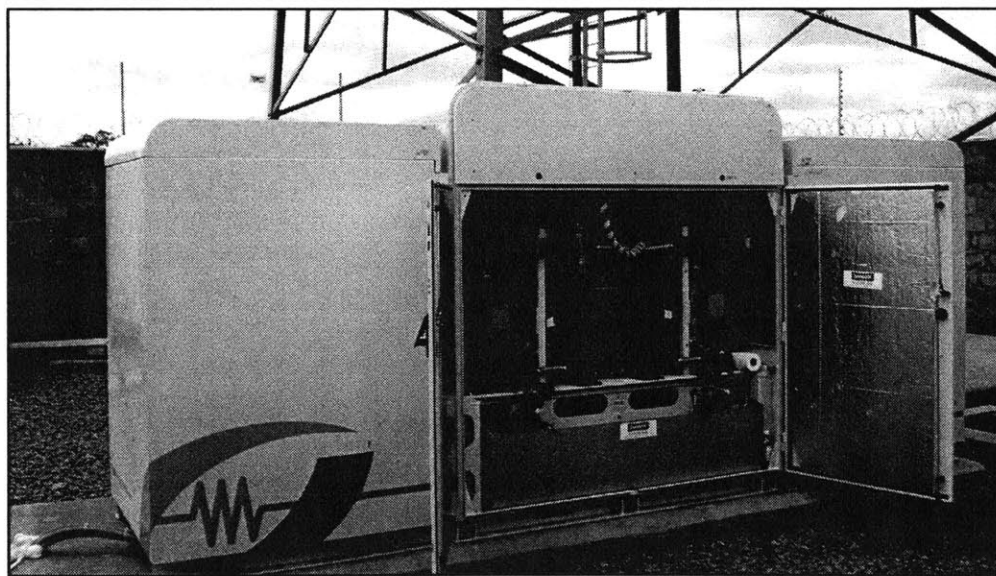
Figure 17: Typical kW-Class VRB-ESS Installation, Njambini, Kenya
