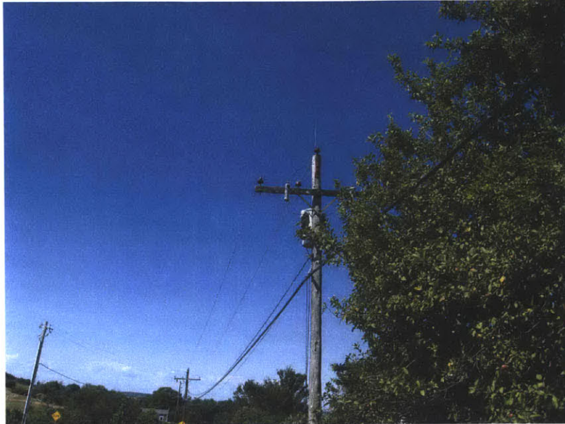
Figure 3.2: Typical Distribution Lines
