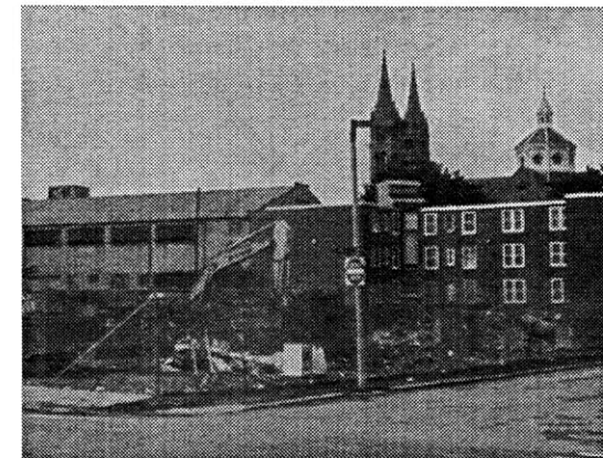
Figure 43: Phase 1A demolition has already begun at corner of Parker and Smith Streets.
