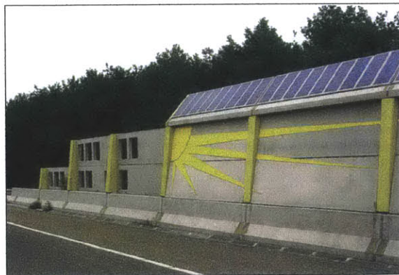
Figure 3.6 A concrete noise barrier painted with the image of the sun and photovoltaic panels on top. Source: Environmental Noise Barriers
