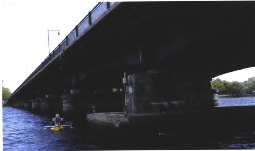
Figure A-4: Our model does not include the pier shown in the foreground near the robot. Original blueprints show a drawbridge, which was removed in 1924. Blueprints of the replacement pier are unavailable.
