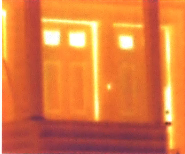
Figure 21: Infrared image of door crack loss
