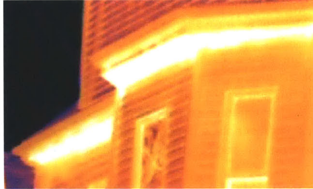
Figure 25: Infrared image of soffit loss
