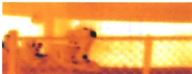
Figure 20: Infrared image of basement loss
