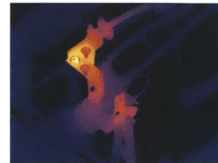
Infrared inspection helps to detect overheating parts, can avoid costly downtime and maintain plant efficiencies.
