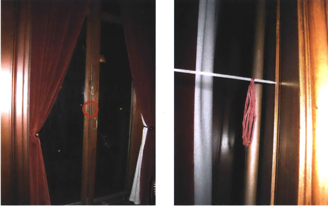
Figure 11: The large windows on the second floor of 478 Commonwealth had substantial cracks, but when the thread tool was used there was no indication of air flow because of the neutral pressure plane.
