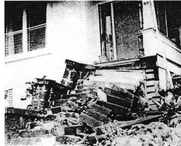
Lava rock foundation wall and concrete stair failure (Robert I. Tilling 7)
