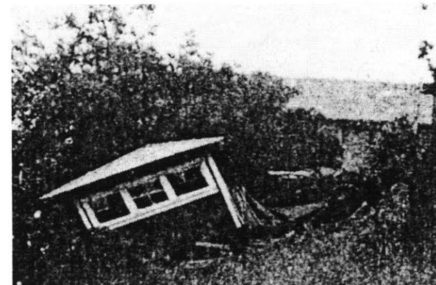
Top: Demolished home Punaluu Hawaii caused by earthquake related tsunami 1975 (Robert I. Tilling 13) Bottom: Post-and-footing failure caused total collapse of the structure (Gordon A. Macdonald & Wentworth 275)
