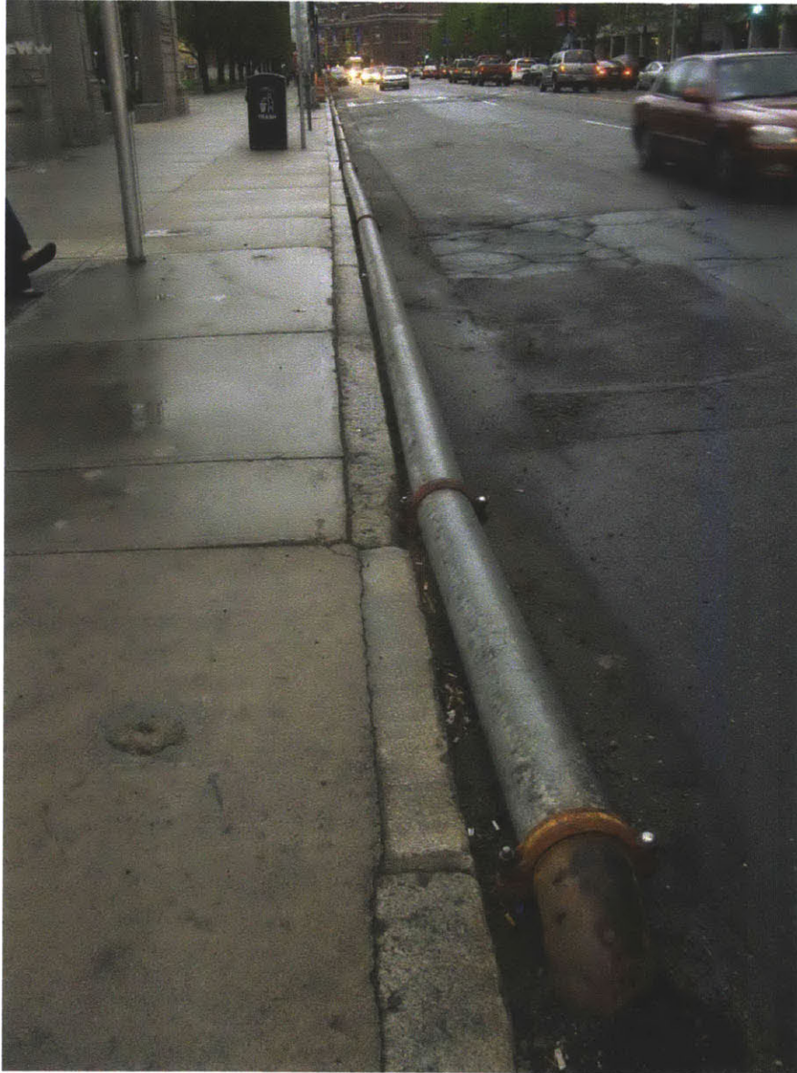
Figure 62 Iron pipe embedded in the street on Massachusetts Avenue (near the Berklee School of Music), Boston, MA. 2011. Photo: Tomashi Jackson
