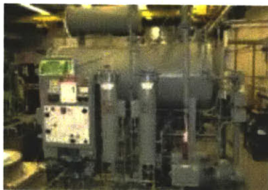
Figure 17: Oil processing unit (OPU) in the pilot area was identified as an opportunity for insulation
