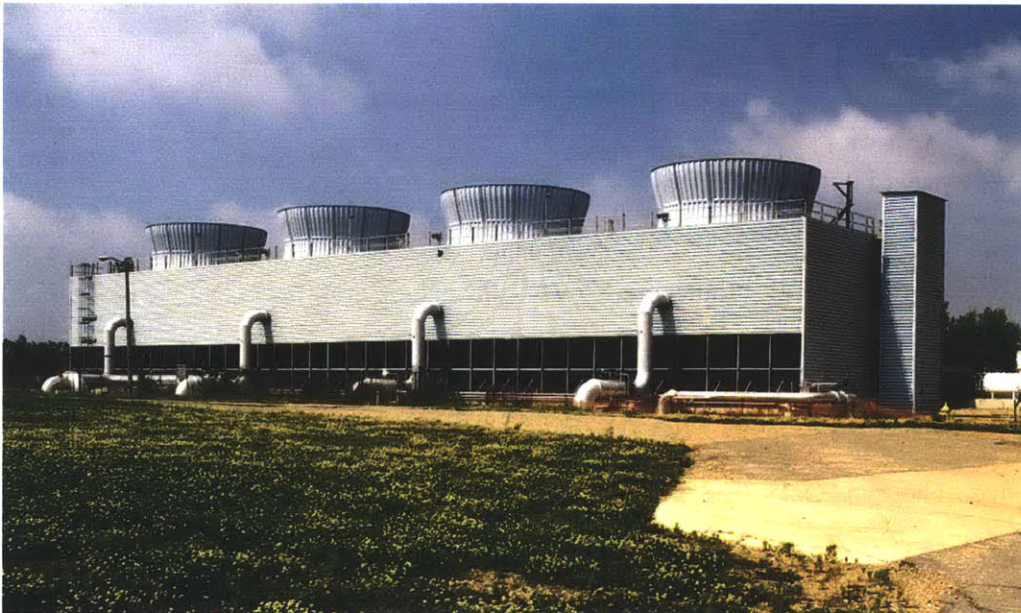
Figure 15. Counterflow Cooling Tower 23
