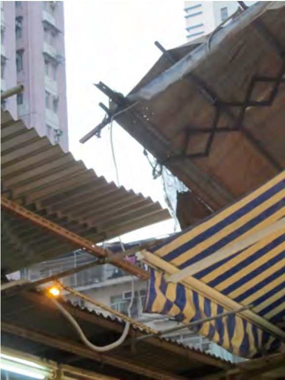
Figure 6: Improvised wiring for vendor stalls
