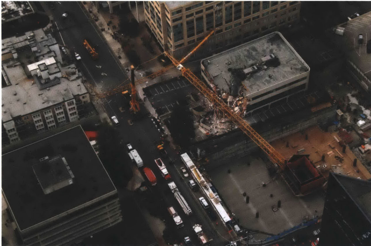
Figure 1.2: A tower crane collapses in Bellevue, Washington. (Haag Engineering Co.)
