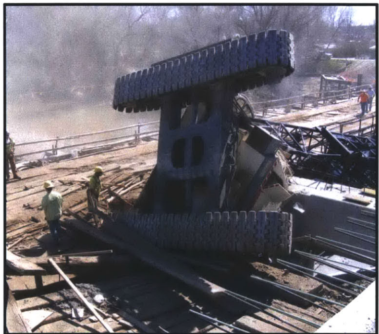
Figure 1.1: Crane stability failure after crawler punches through a surface. (Haag Engineering Co.)
