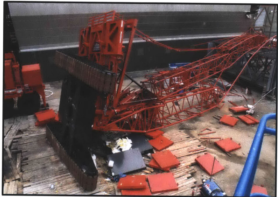
Figure 5.2: Stability failure of a mobile lattice crawler crane. (Haag Engineering Co.)
