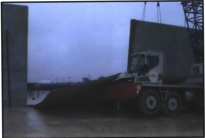
Figure 5.3: Tilt-up wall falls on crane during erection. (Haag Engineering Co.)
