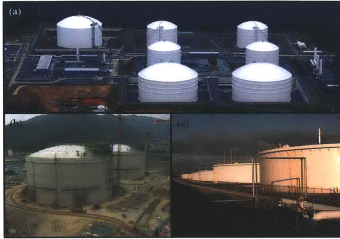
Figure 1-1: LPG Storage Tanks. (a) Dominion Cove Point LNG facility located in Lusby, Maryland. Photo courtesy of Dominion Corporation [1]. (b) Two LPG storage tanks. Photo courtesy of Lusas Corporation [2]. (c) Row of LPG storage tanks. Photo courtesy of Gauging Systems Inc [3].
