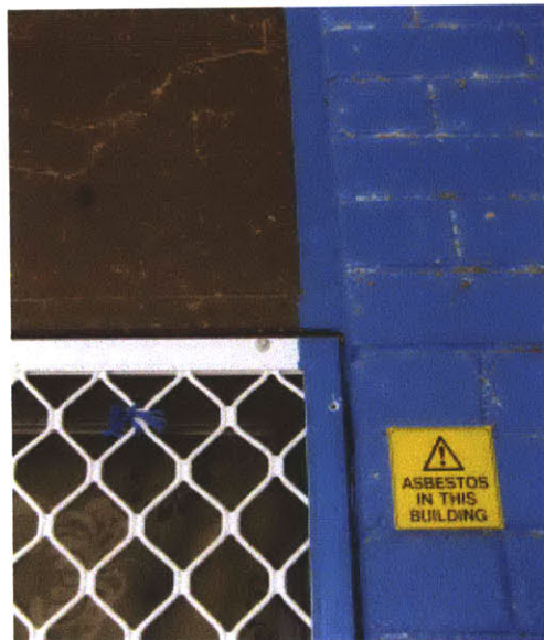
Figure 13: Asbestos in Residential Buildings, Beswick
