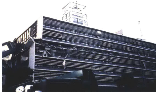
Figure 1.4.1. Mid-story failure of Kobe city hall from the 1995 Kobe earthquake.
