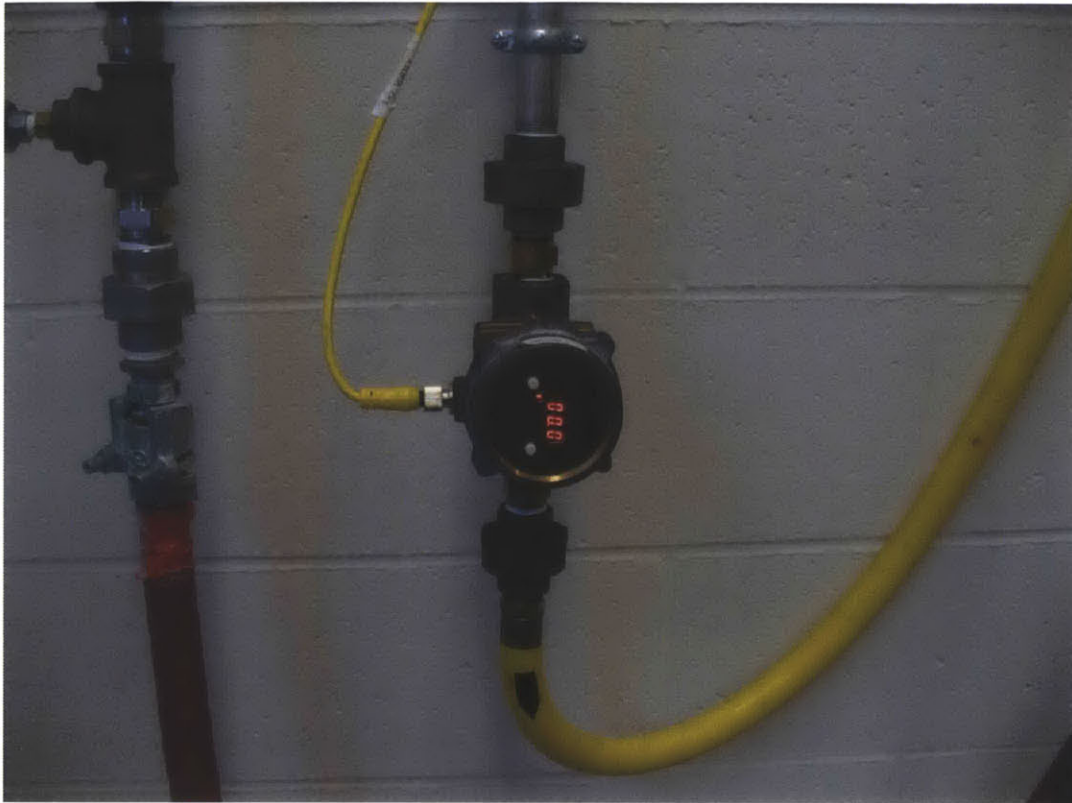
Figure 6-34: Photo of Vortex Flow Meter
