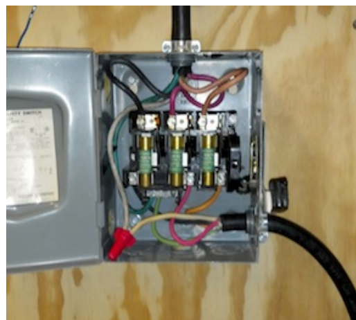
Figure 2-2 Emergency Shut-off Switch
