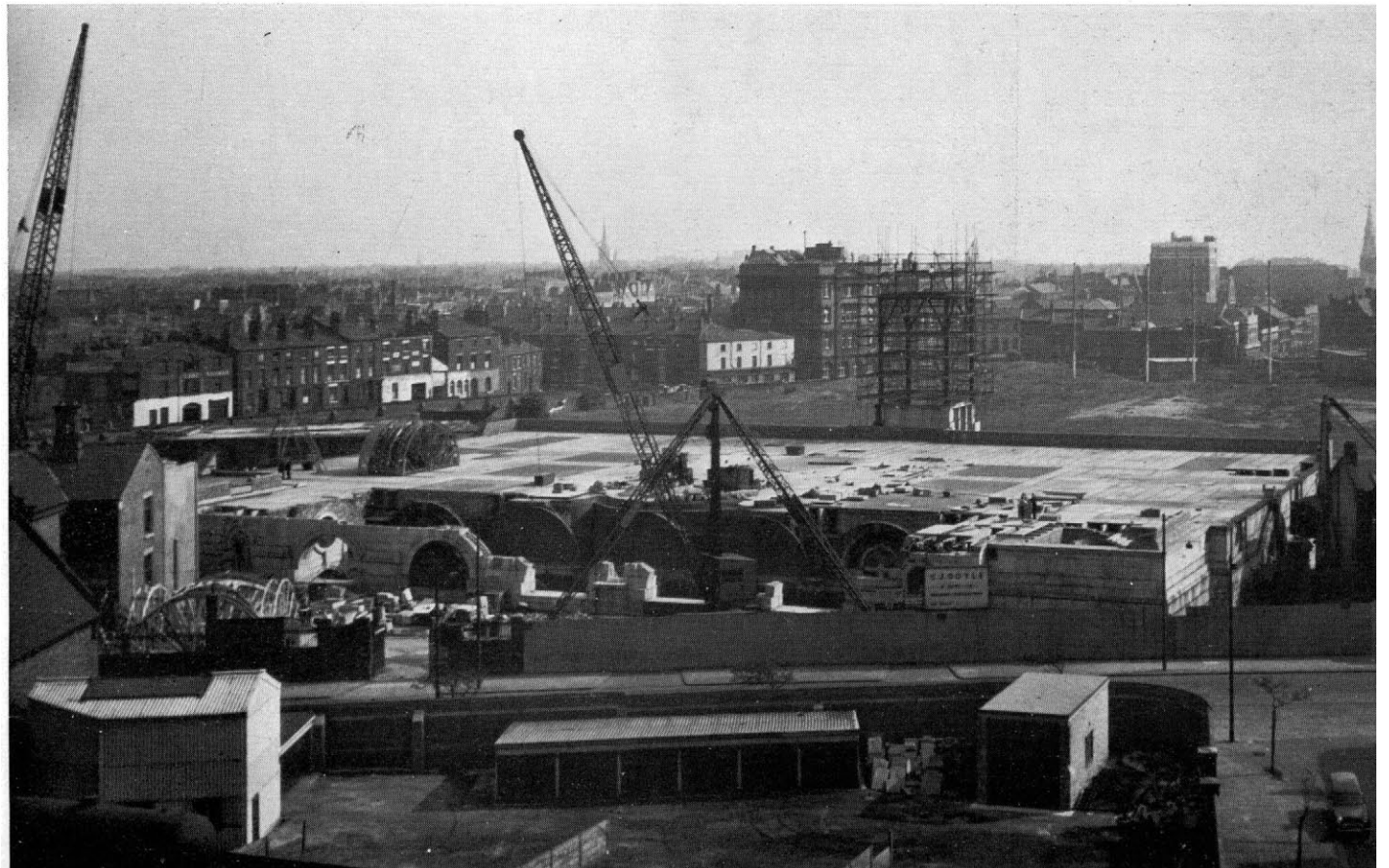
Looking south over roof of crypt (still under construction), with temporary altar beyond. Brownlow Hill runs across the picture in the foreground.
