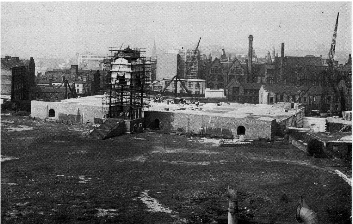
Site from southernmost point looking north, showing south wall of crypt and temporary altar (in scaffold).
