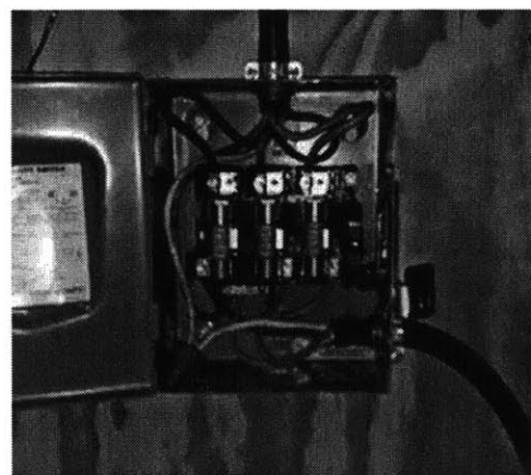
Figure 2-2 Emergency Shut-off Switch
