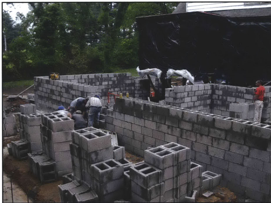
Figure 86. Concrete blocks are often used for perimeter walls in construction, as seen here. Image source: Home Designs and Furniture Gallery
