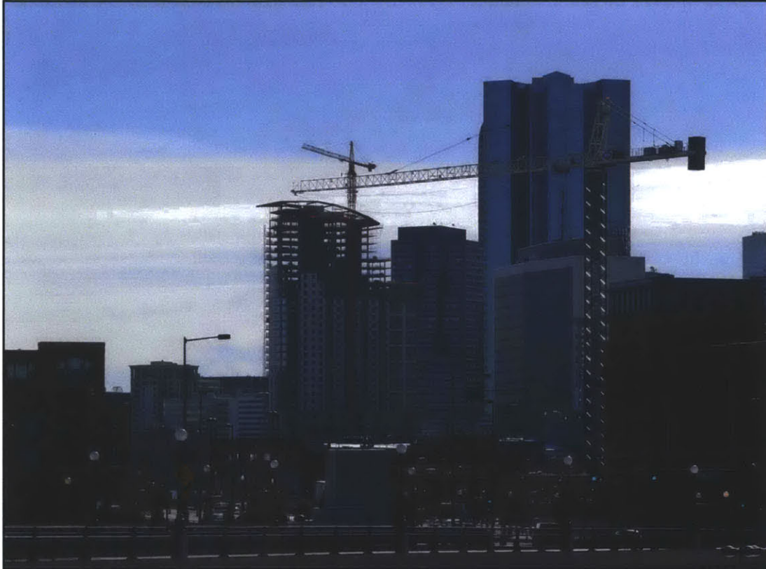
Figure 87. Large skyscrapers are constructed using a backbone of steel. Image source: Denver Infill Blog
