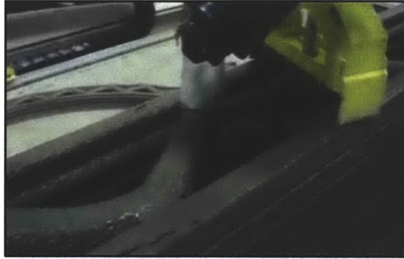
Figure 62. The Contour Crafting project uses a direct extrusion process combined with a trowelling process to additively create large concrete structures, like the wall seen here. Image source: Contour Crafting, University of Southern California
