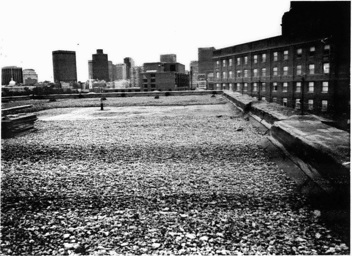
Existing roof today, with Edge Encapsulation visible. Note the pipe and wire railing detail.
