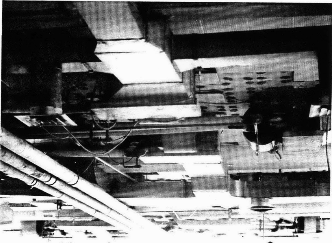
Antiquated Ventilating and Air-Conditioning System
