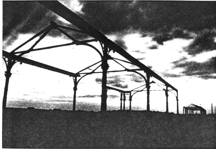
Pavillion at mid-beach, missing roof due to 1978 blizzard, but shape of iron frame clearly visible.
