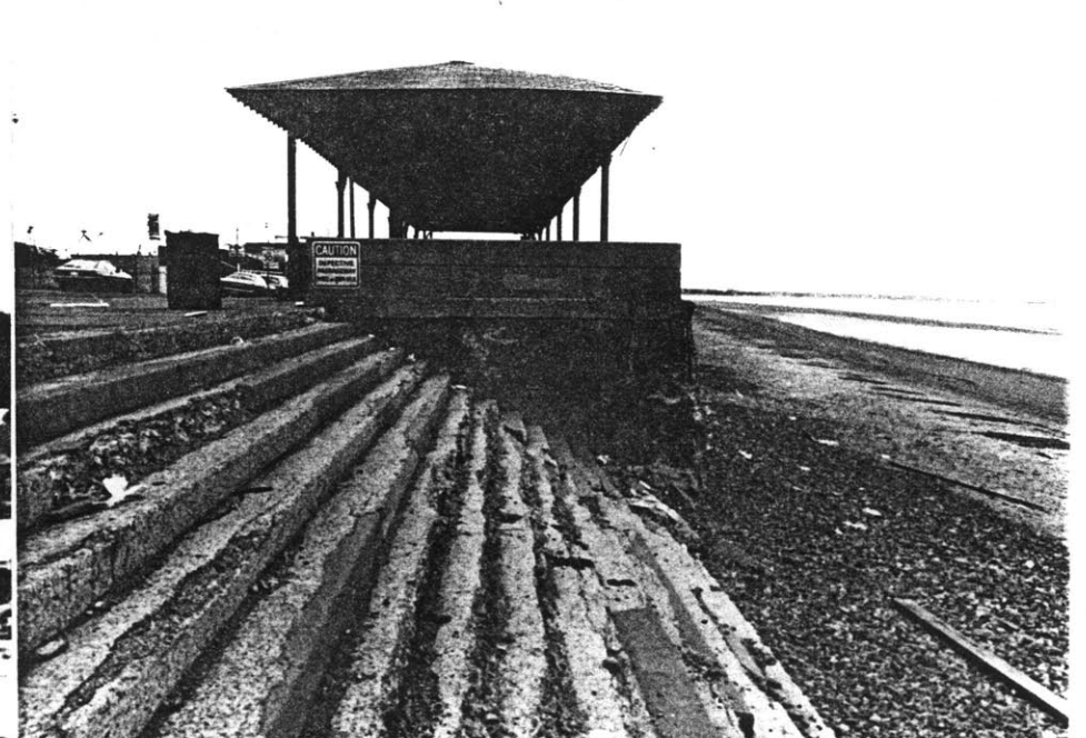
Steps and seawall in disrepair. Sand eroded from beach.
