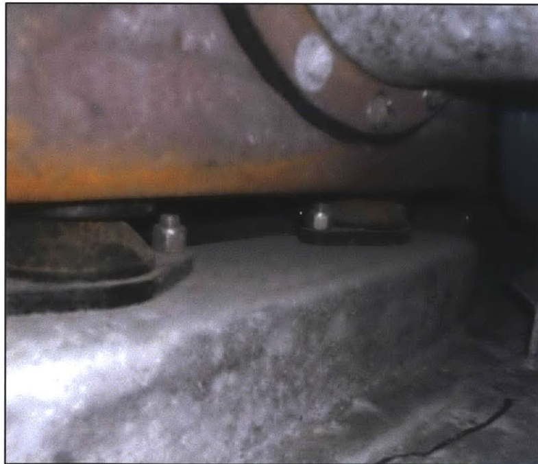
Figure 70: Side View of Vibration Mounts on SENECA.
