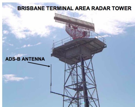
Figure A-4: Temporary Installation of an ADS-B Antenna on a Terminal Area Radar Tower in Brisbane, Australia (credit: Greg Dunstone)
