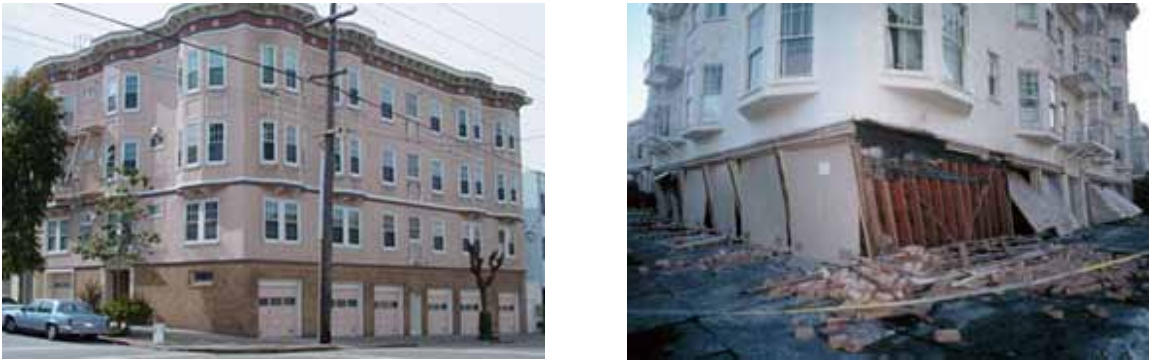
Figure 4.1.1. Wood-frame soft-story corner building (left). Effects of seismicity on soft-story (right). Image courtesy of Association of Bay Area Governments.
