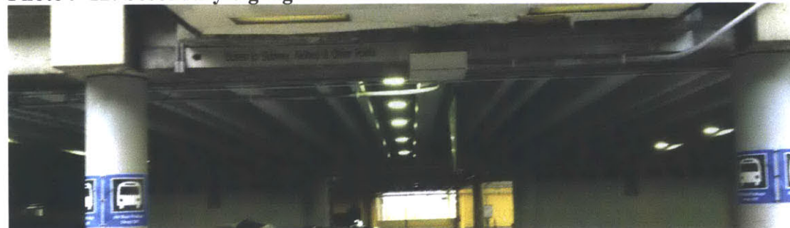
Photo 9-13: Outdated Curb Signage, Terminal B-East
