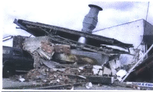
Figure 1-8: Destroyed structure, Christchurch 2011
